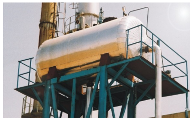
Pic. Pressurized Steamline deaerator at Fresenius Kabi, Ranjangaon
